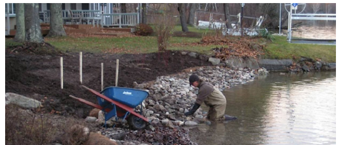
Biotechnical erosion control project being installed at a higher energy inland lake shoreline. Photos courtesy of Jennifer Buchanan, Tip of the Mitt Watershed Council.
