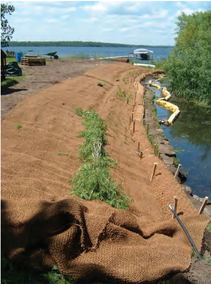
Figure 4.15. Wattles staked in to secure ECBs at their overlap. Notice how the upper blanket overlaps the lower blanket. (Photo: Jane Herbert.)
