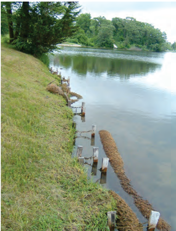
Figure 6.2. Poorly maintained coir logs can become a navigational hazard when displaced by wave action. (Photo: Jane Herbert.)
