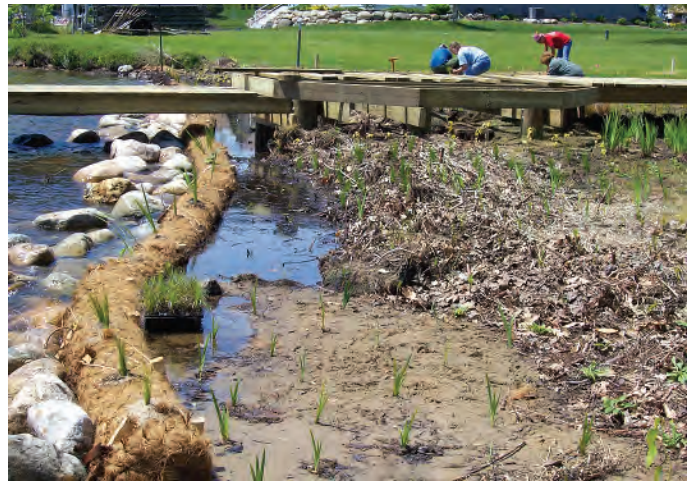
Figure 4.26. Planting native wetland plants in and behind the coir logs (May 2005). (Photo: JFNew.)
