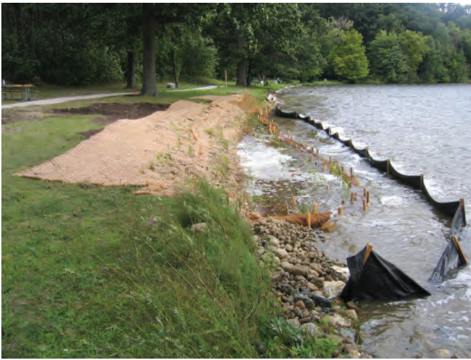
Figure 4.14. Coir logs of insufficient diameter are overtopped by waves, which then disturb nearshore aquatic plantings. (Photo: Jane Herbert.)
