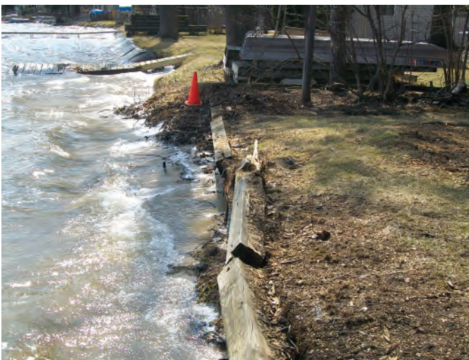
Figures 4.18. “Before” picture of a failing wooden seawall, (Photo: Jane Herbert.)
