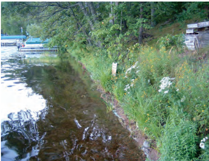
Figure 4.12. Undercut bank stabilized with a biodegradable log (brush bundle) and plantings. (Photo: Jane Herbert.)
